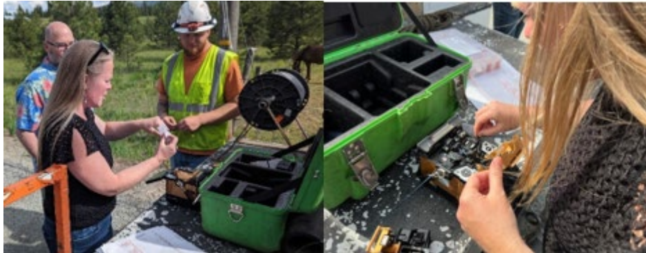
Figure 5. IOB Project Manager Krista Baker on a MiFiber site visit learning how to splice fiber in the field.
